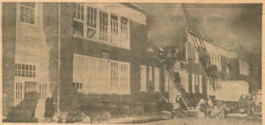
BREAKTHROUGH. Firemen scramble up ladder toward opening smashed in wall by crane's bucket, behind ladder on ground, at Bellport school fire yesterday. Opening enabled firemen to play hoses directly on blaze.
