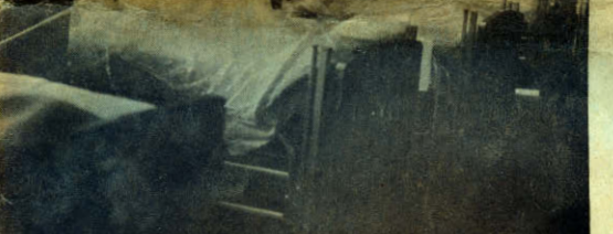
REPAIRS on the center two-story wing, with possible other damage yet to be determined.
