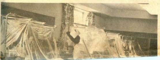
REPAIRS on the center two-story wing, with possible other damage yet to be determined.
