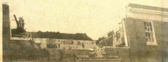
MAIN WALL of Bellport Junior-Senior High School fronting on Station Road was knocked down by Brookhaven National Lab's crane to permit firemen to get at fire more easily.
